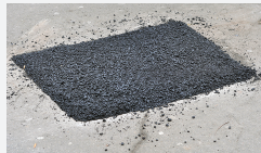
Temporary asphalt repair patch in street and/or sidewalk after service line replacement.
